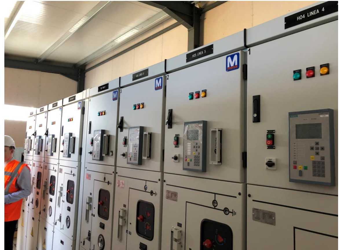
Medium voltage switchgears
