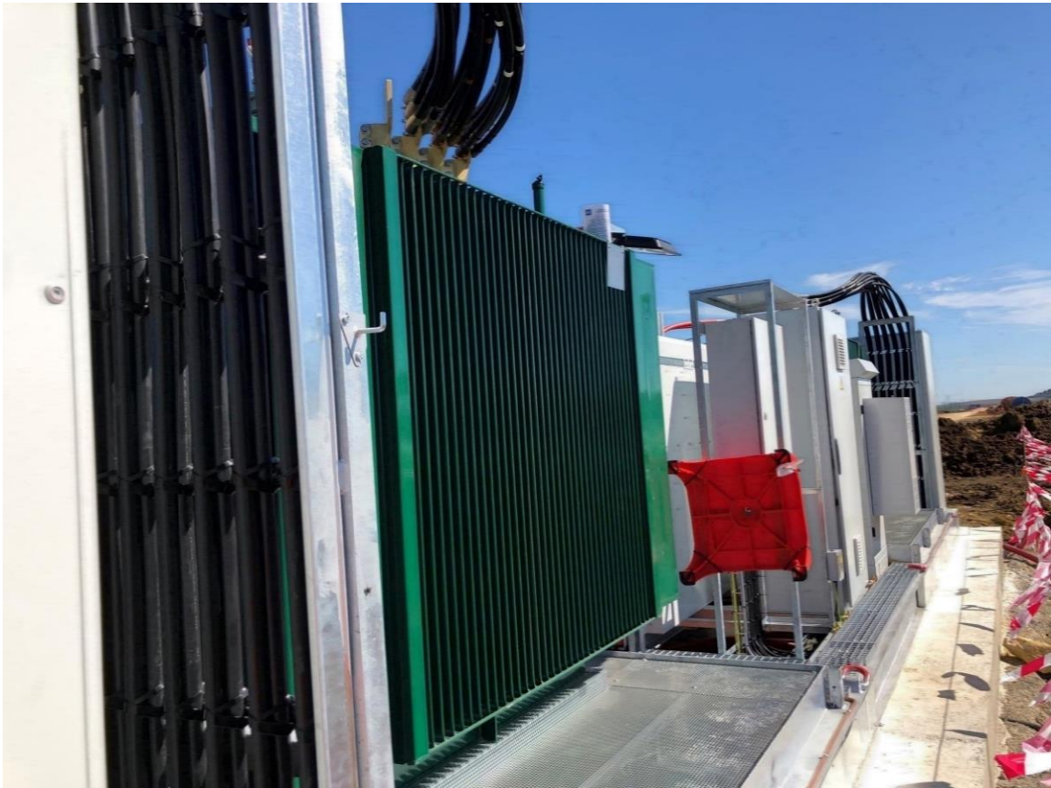
Low voltage/medium voltage transformation platform
